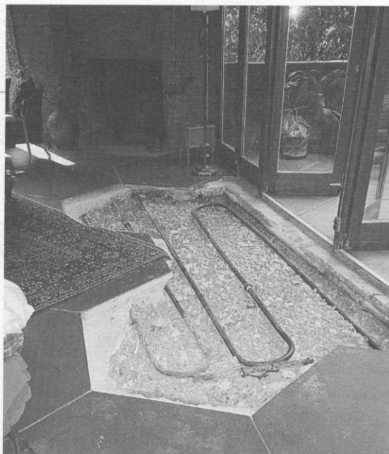
Final repair after (3) hex. units and (2) half hex. units of concrete were removed to repair additional deteriorated pipe.
